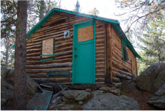
Figure 3.7. The only true log building inventoried as part of the survey, this cabin on Olde Carter Lake Road (5BL.11028), has hog-trough corners with decorative log cornerposts. (Photograph by Adam Thomas.)
