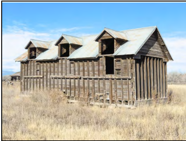
A rare studs-out granary with dormers, which were used for filling the building with grain. Photo by Carol Beam, BCPOS.
